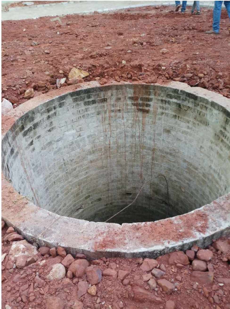
Structure of Recharge pit
